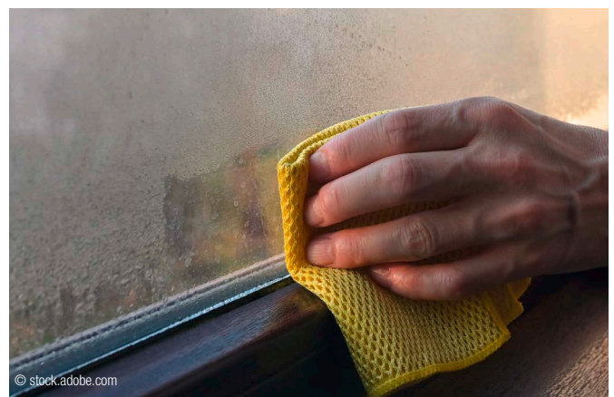
Condensate on the inner side of the window
